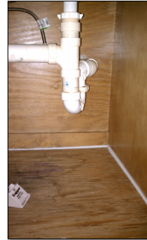
Monitor under a well-sealed sink
